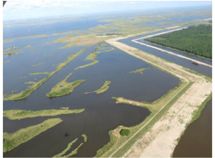
Aerial view from the southeast looking towards the northeast section of Catfish Lake. The project will hydraulically dredge material from the lake to restore the fragmented marsh along the lake rim.
